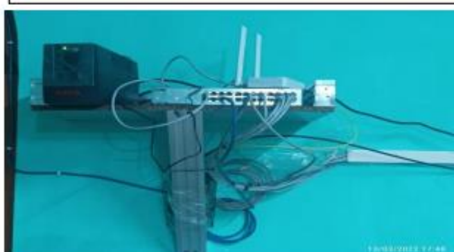
High Speed Optical Fiber Internet Connection
